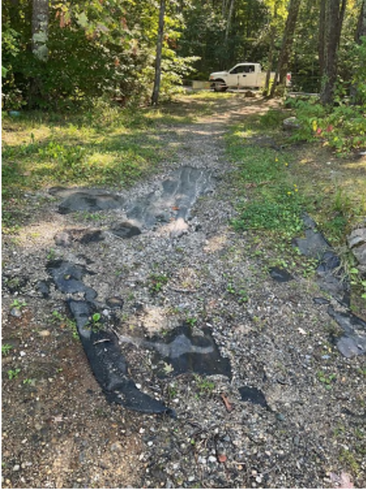
Figure B-39 Erosion at The Basin Access Point Near UB-4
