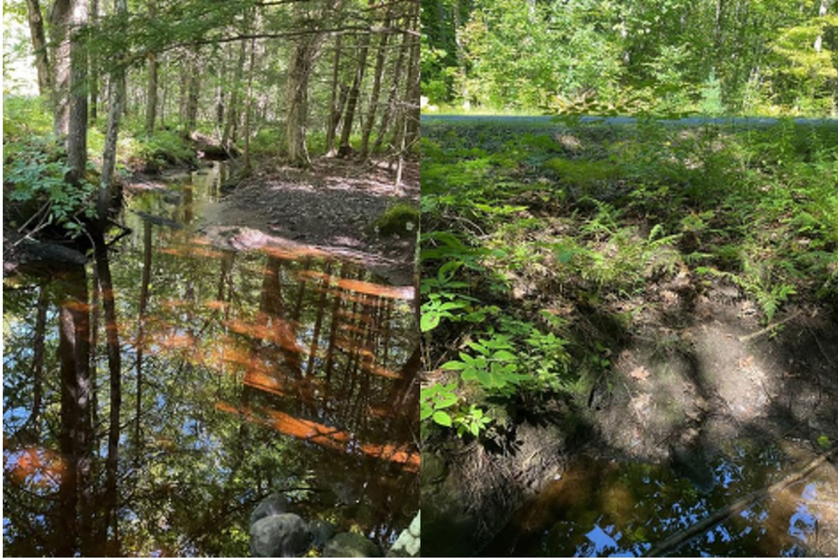
Figure B-48 Erosion Upstream and Along the Roadside on the Wilson Hill Road Culvert (Turner)
