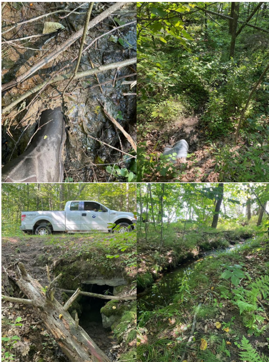
Figure B-32 Examples of Typical Erosion Patterns in Culverts on Whitman Spring Road Clockwise from top left: silty clay sediment accumulation upstream; partially collapsed culvert with sediment accumulation downstream; significant outlet erosion; undercut bank downstream of culvert
