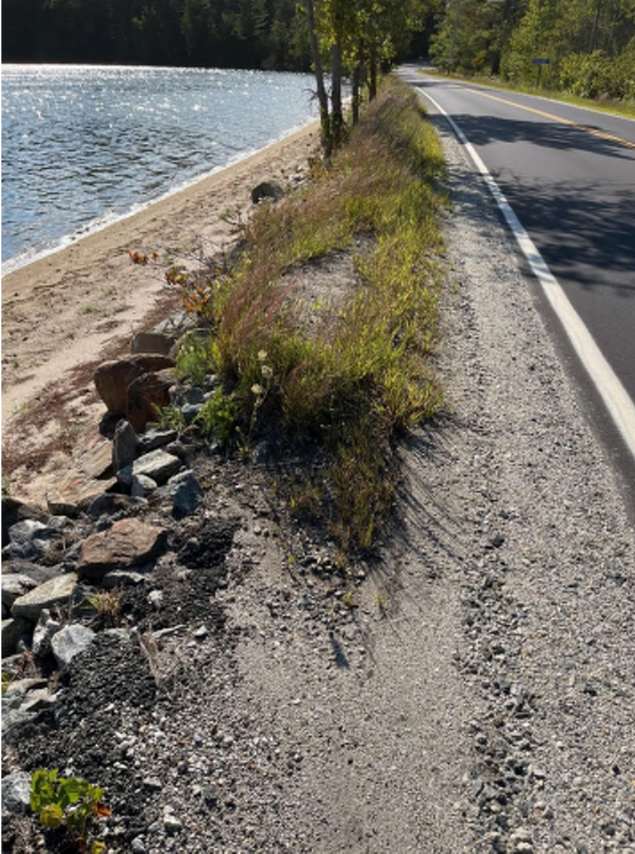
Figure B-21 Shoreline of Lake Shore Drive Showing Vegetated Filter Strip with Gap Causing Erosion to Reach the Lake
