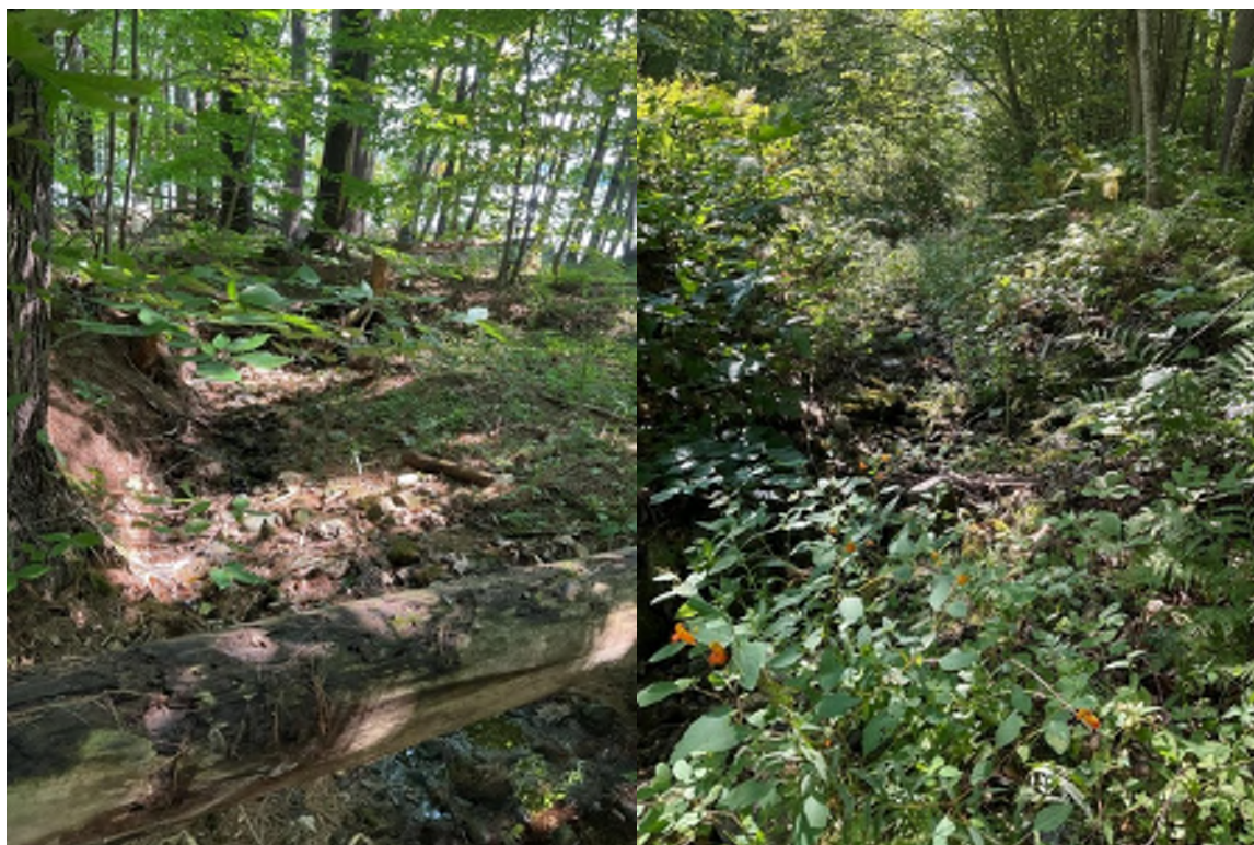
Figure B-30 New Culvert at location SR-3 with Evidence of Significant Downstream Erosion (L) but Well Armored Upstream (R)
