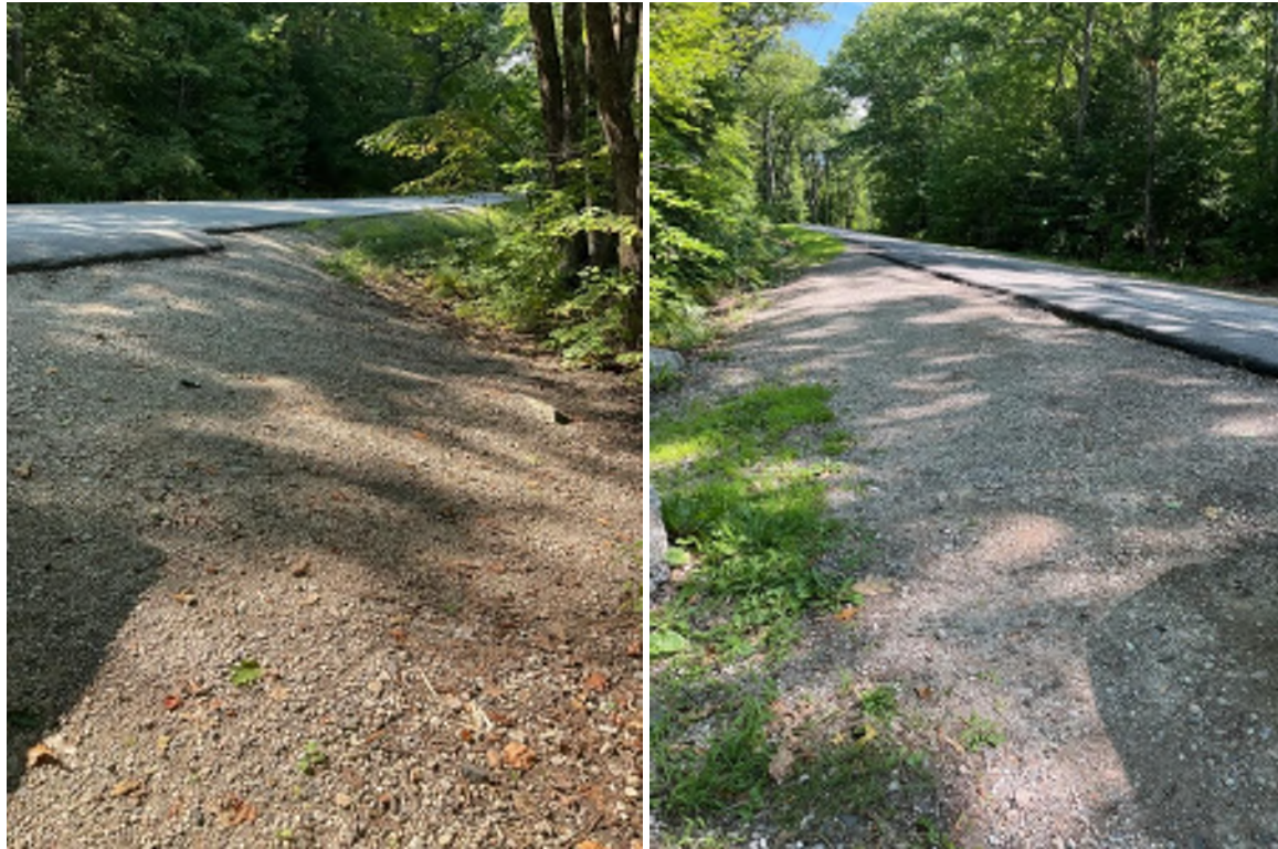
Figure B-38 Erosion at Gravel Parking Areas on Holbrook Road near the Basin
