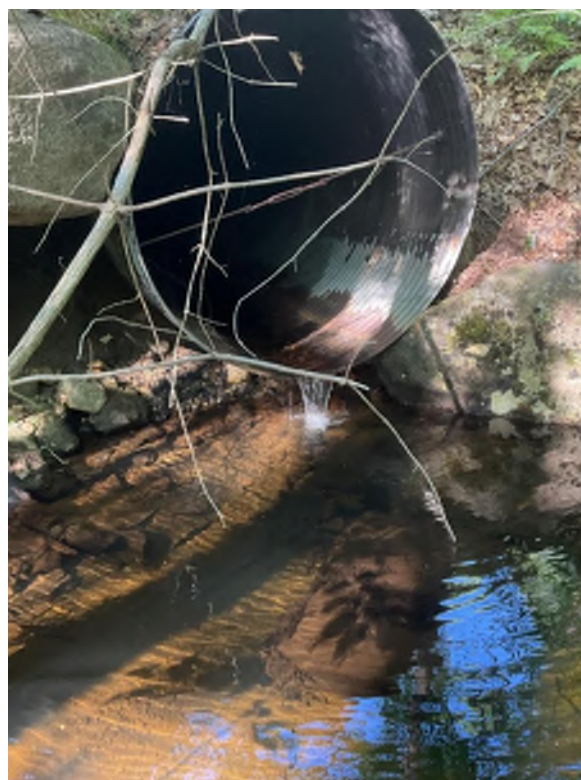
Figure B-6 Sediment in the Pool Underneath the Culvert Crossing at Lake Shore Drive
