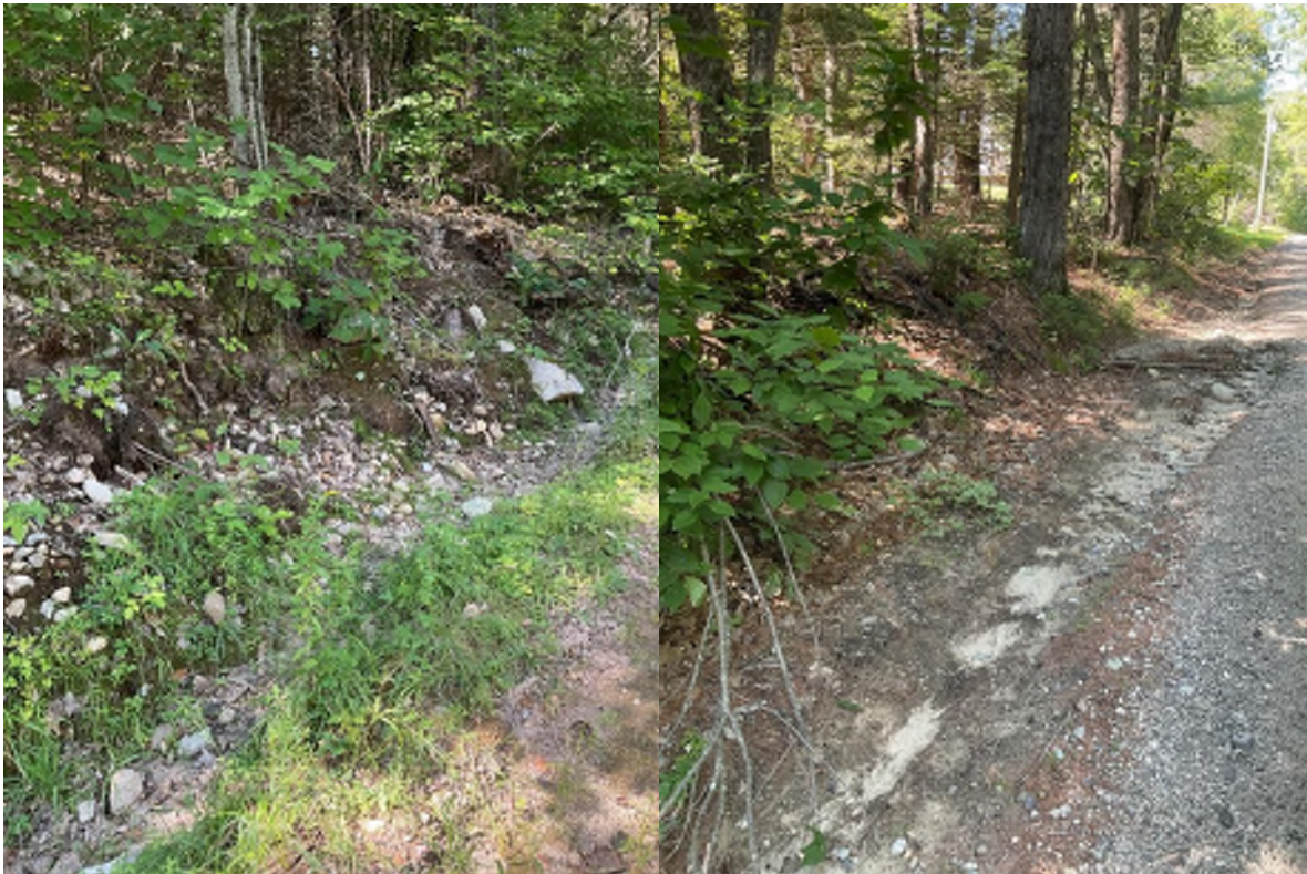
Figure B-53 Erosion on Boutin Road and Adjacent Steep Slopes
