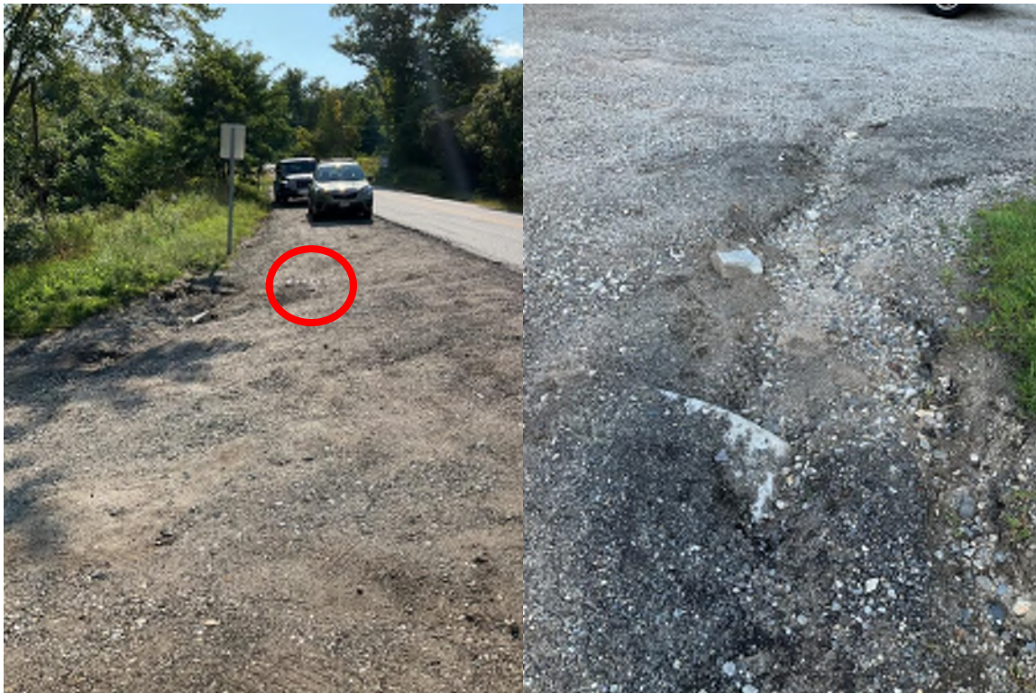
Figure B-27 Eroding Parking Area and Catch Basin at Northern Whitman Spring Road Parking Area
