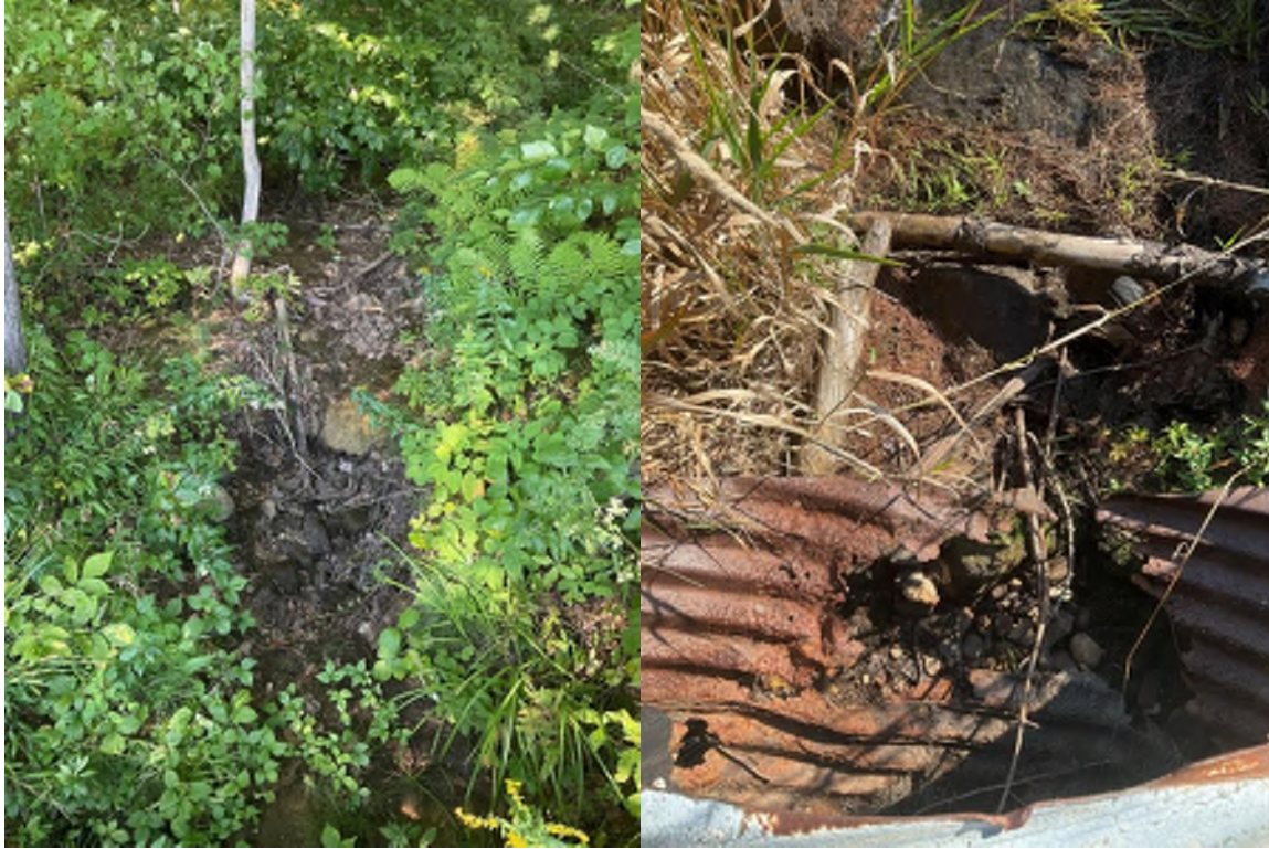
Figure B-10 Erosion on Steep Stream (L) and Culvert in Poor Condition (R)
