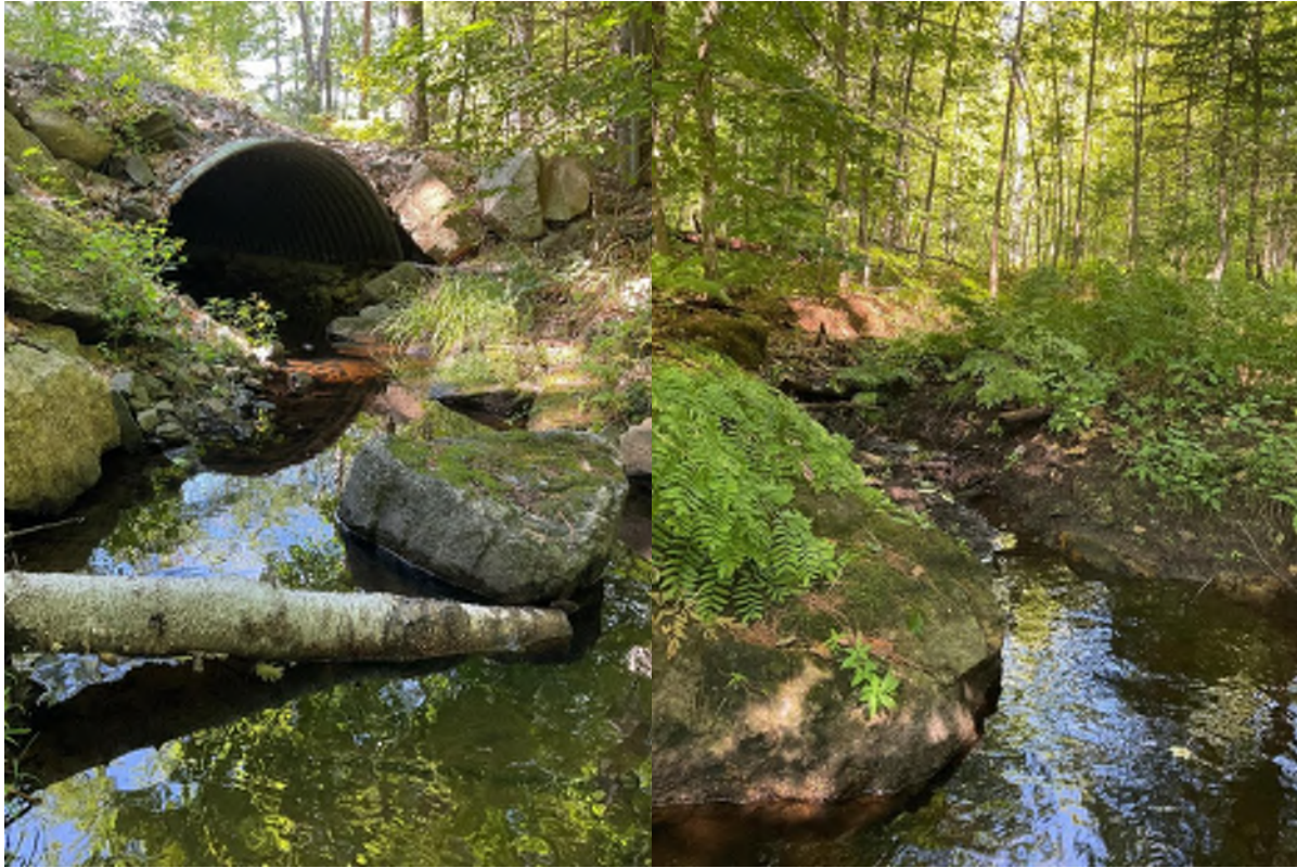
Figure B-50 Replacement Culvert at Little Wilson Pond Road with Significant Sediment Accumulation
