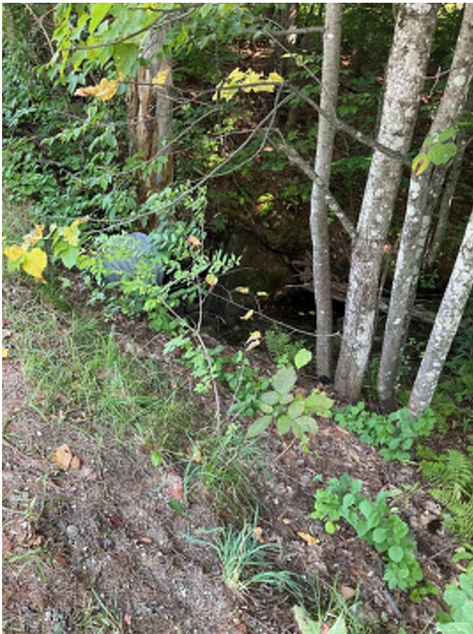
Figure B-47 Erosion at Outlet Embankment on Bailey Road Culvert
