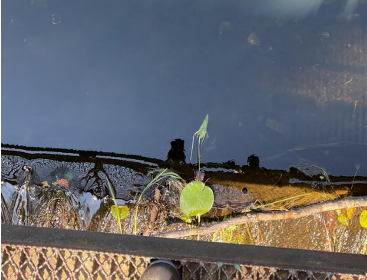
Figure B-36 Sediment Accumulation at the Basin Dam
