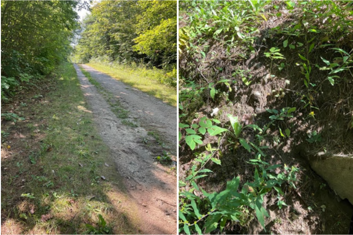
Figure B-29 Slope at SR-4 and Erosion on Culvert Outlet Embankment
