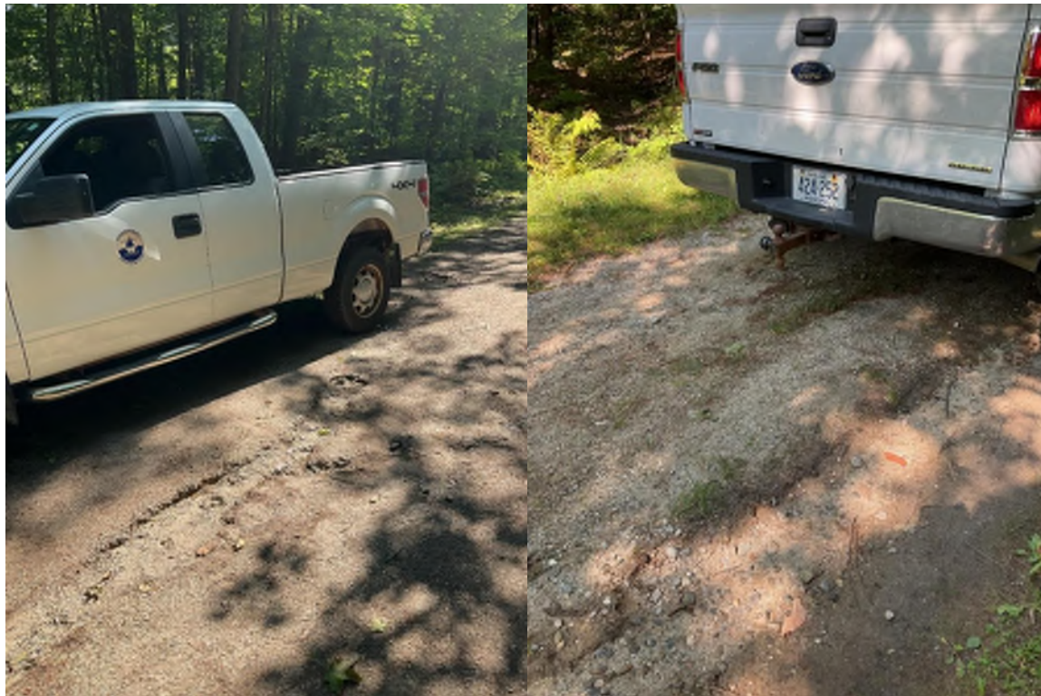
Figure B-28 Erosion on Surface of Whitman Spring Road
