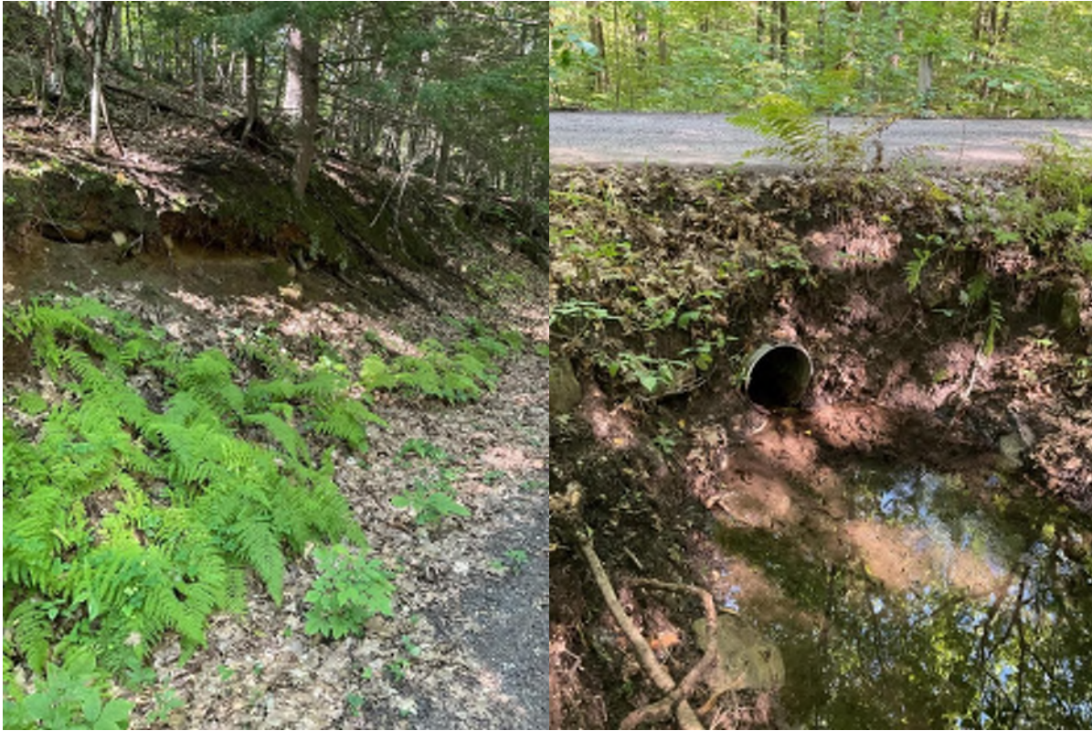
Figure B-51 Robinson Road Erosion
