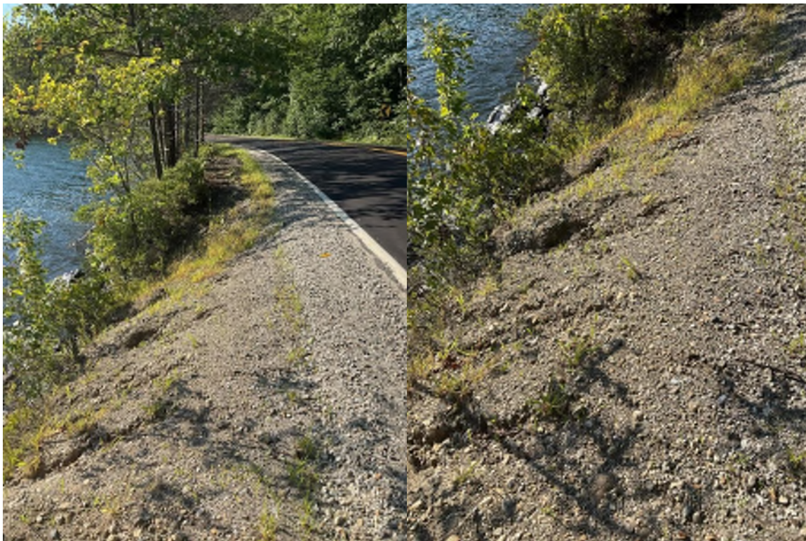
Figure B-8 Vegetated Buffer on Lake Shore Drive (L) and Erosion (R) Note erosion in foreground leading to the lake
