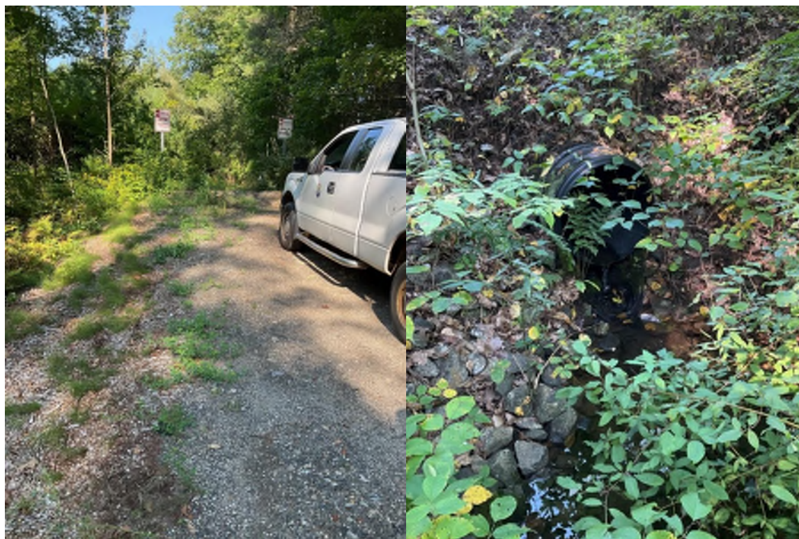
Figure B-34 Erosion from Snowplow Turnaround (L) and Erosion at Culvert Outlet (R)
