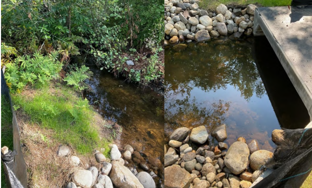
Figure B-14 Erosion in the Stream Near Tot Lot Culvert (L) and Recently Replaced Tot Lot Culvert ®
