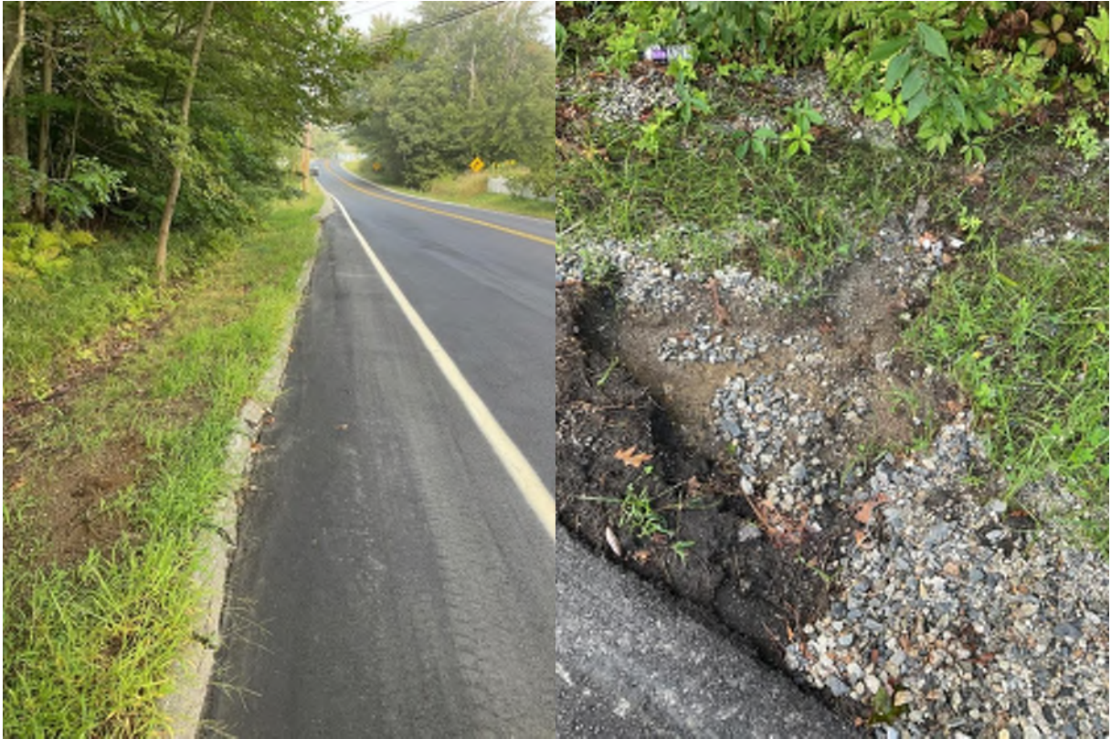
Figure B-23 Erosion on the Lake Side of Lake Shore Drive at the Route 4 Intersection
