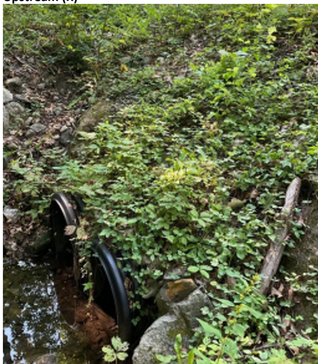
Figure B-31 Culvert at SR-3 with Significant Embankment Erosion
