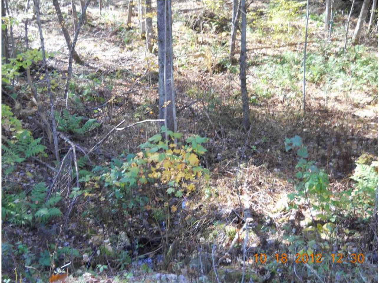
Steep forested slope leading to 24 inch roadside inlet. Outlet has scoured channels
