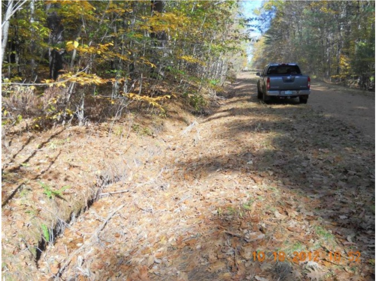
Eroded roadside flowing south to box culvert inlet at bottom left
