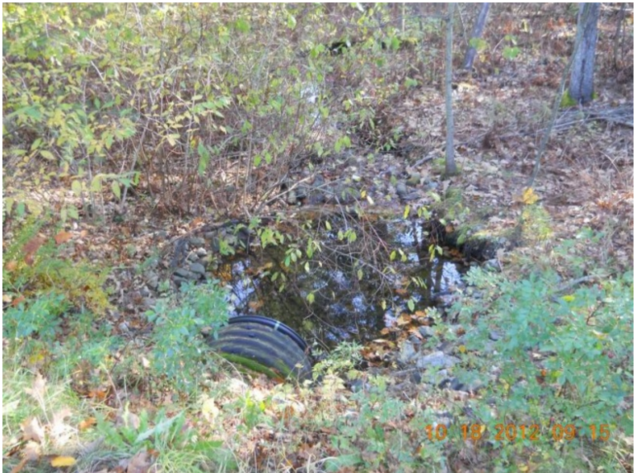
Armored 30 inch HDPE Inlet. Note accumulated sediment right before standing water
