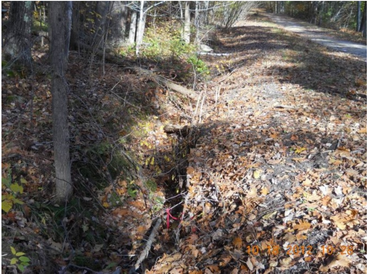
Roadside erosion and partially clogged box inlet. Near a residential house
