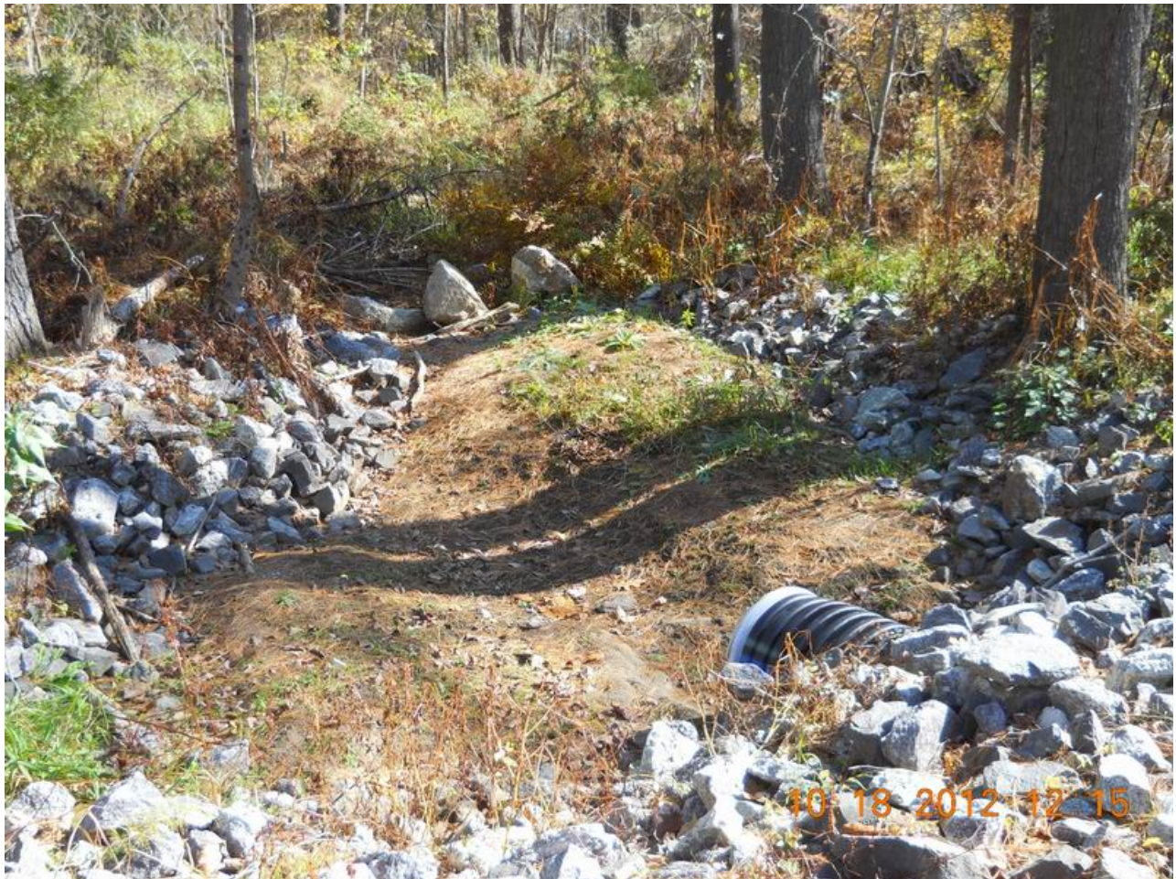
Outlet plunge pool filled with sediment. Inlet also contains heavy sediment deposits
